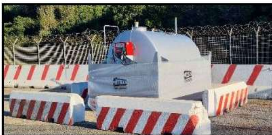
New tank at FCO for HVO storage and supply
