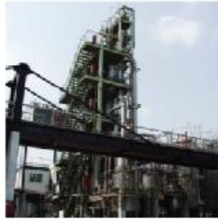
Waste solvent distillation purification equipment
