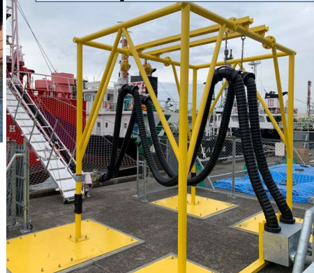
Shore power facilities
