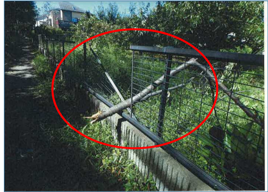
Fallen trees damaging fences on private property
