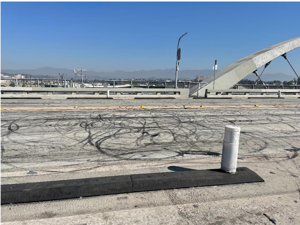
橋面違規特技騎車烙痕(Sixth Street Viaduct)
