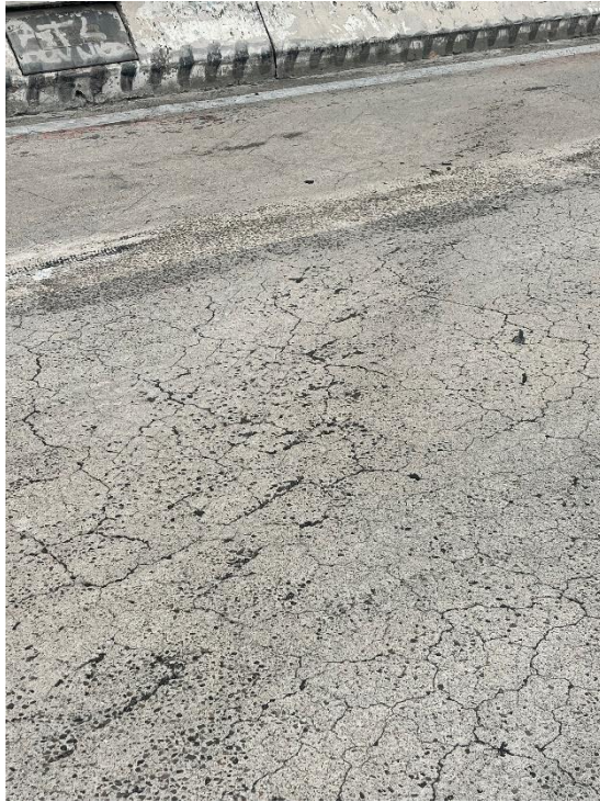
橋面板嚴重裂化(Rio Houdo Busway Bridge )
