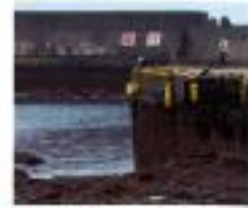
Bridge falling part has been raised by 3 Jan. 3 January 2024
