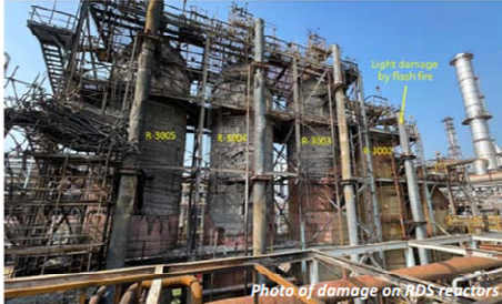
Photo of damage on RDS reactors
