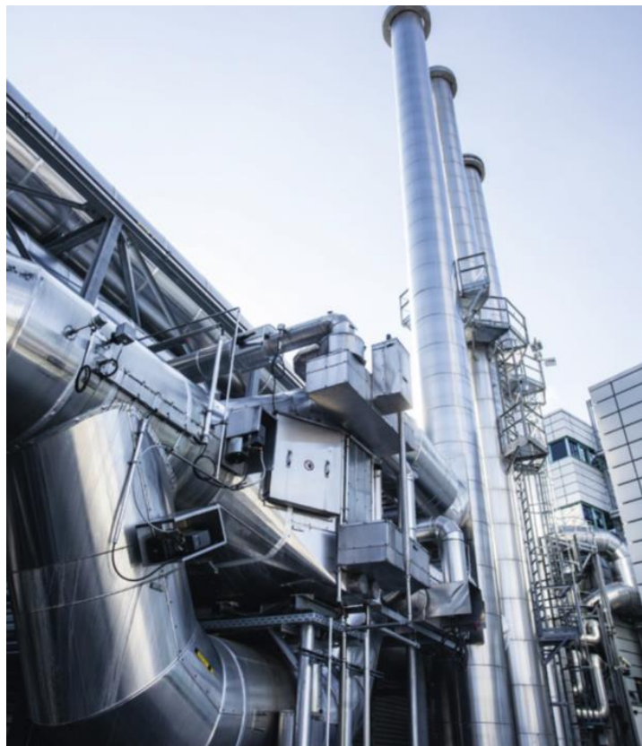
圖 3、汽電共生爐 (combined heat and power, CHP)
