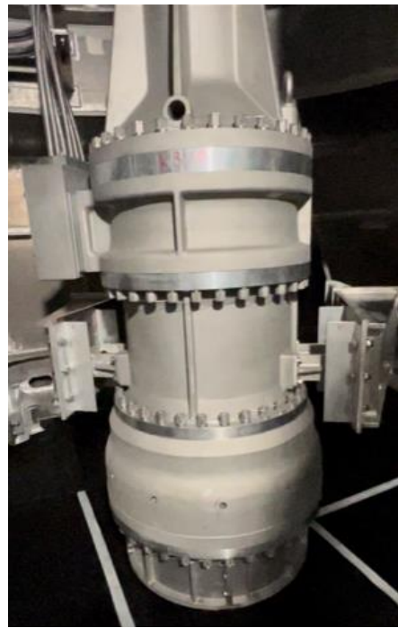
Cargo Pump with strainer (PUMP 下方濾網)
