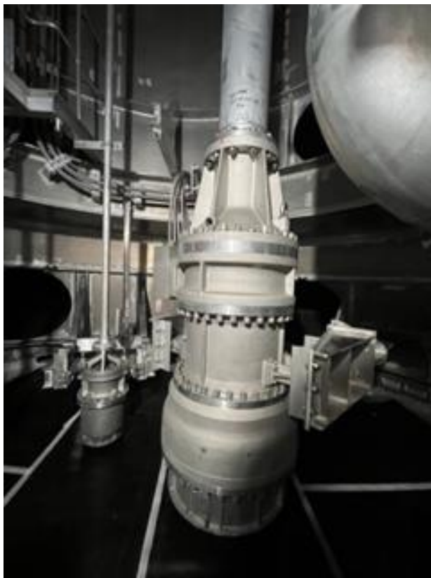
Cargo Pump(圖右)
