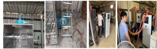
Blower installed in drying box
