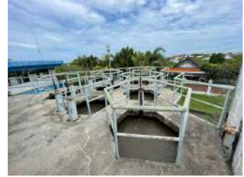
(Coagulation flocculation unit)
