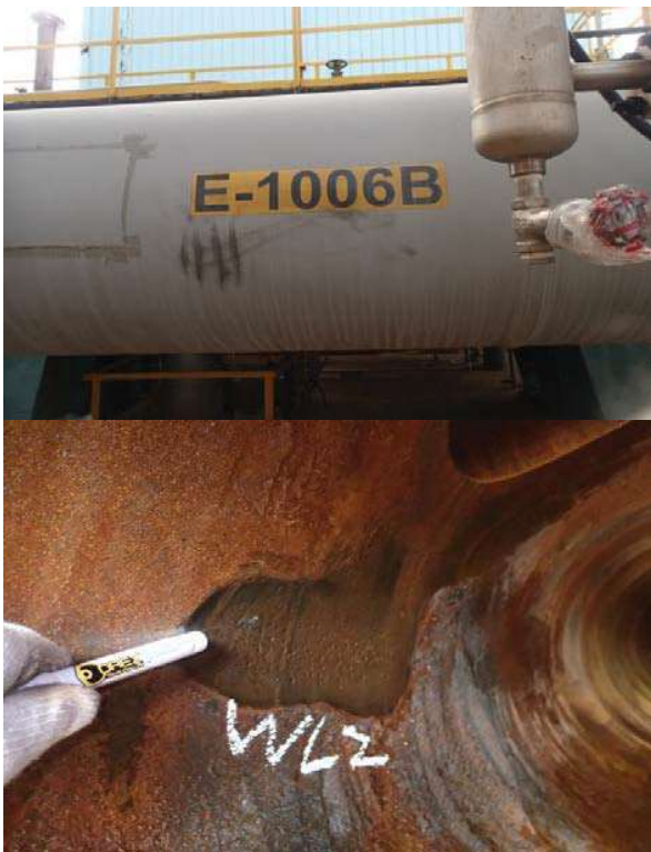
Figure 12: Localized corrosion @ E-1006B S2
