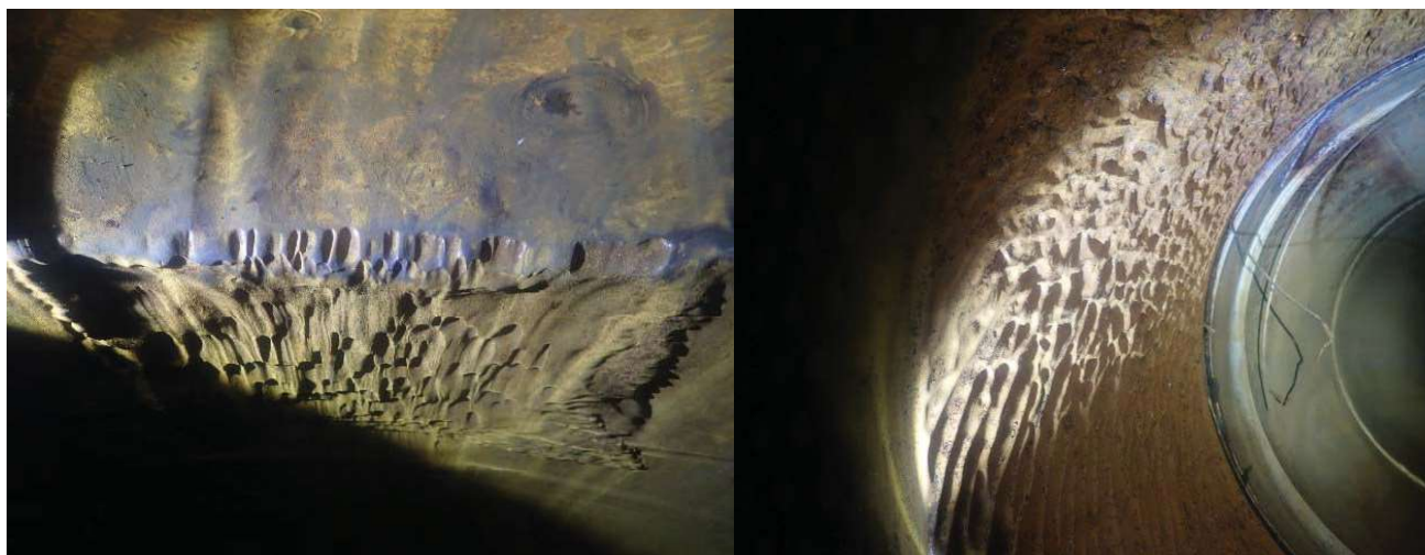
Figure 6: Internal Corrosion Pattern @ D-109 S3
