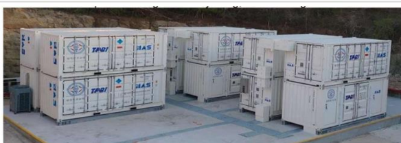
Figure 1. The 1.8MW/10.8MWh long duration application EESS I
