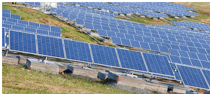
Difficulties with Installation on Slopes (constructability and impact on landfill slope stability)
