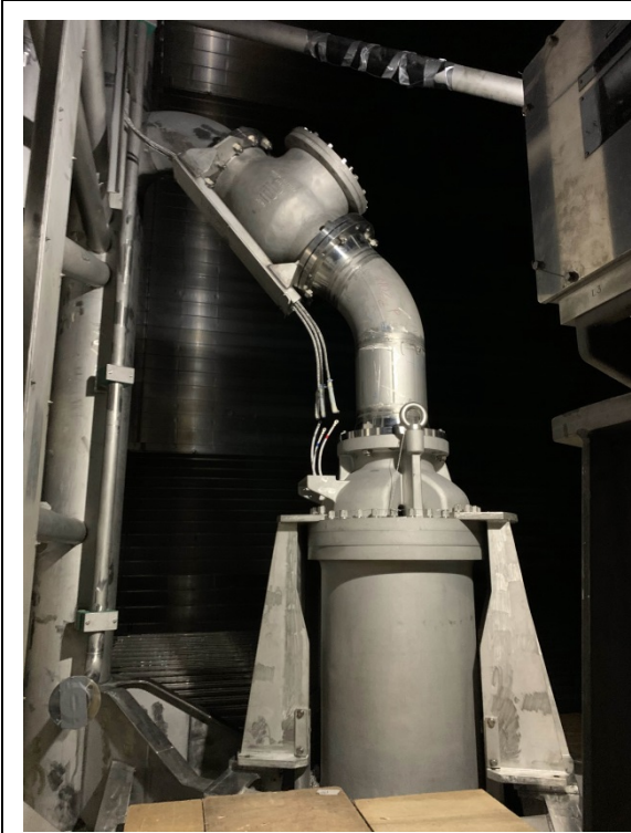
貨艙Cargo Pump及Check Valve
