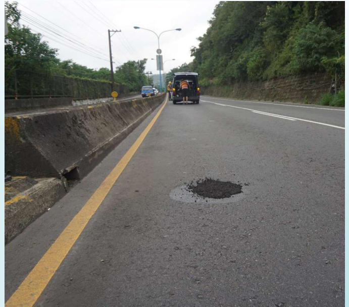
Example of poor patching (Photo taken by DGH)
