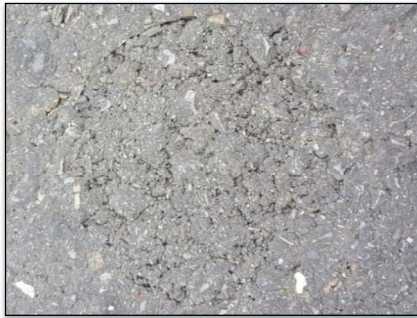
Regular patching materials (After four months)
