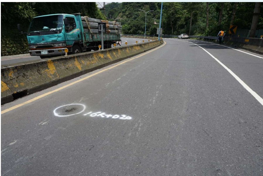
Pothole due to moisture susceptibility (Photo taken by DGH)
