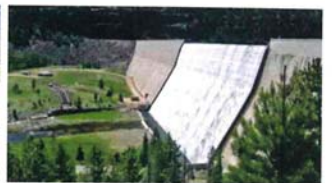
Upper Stillwater Dam - roller compacted concrete gravity dam located on Rock Creek.
