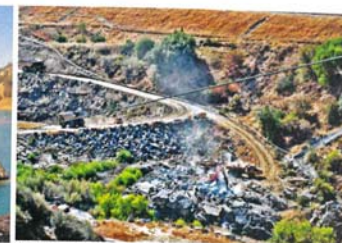
Folsom Dam - currently under construction, a new spillway is the key feature to improving Folsom's flood control ability. When completed, the spillway will operate in conjunction with Folsom Dam's spillway gates to release water earlier during an extreme storm, thus reducing hydrologic risk.
