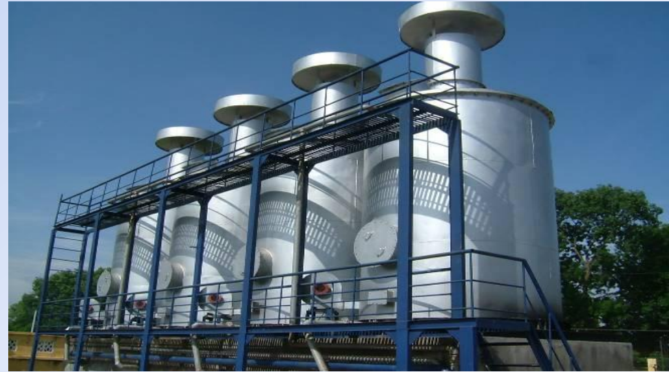
Tuyen Quang General Hospital W.W. treatment system
