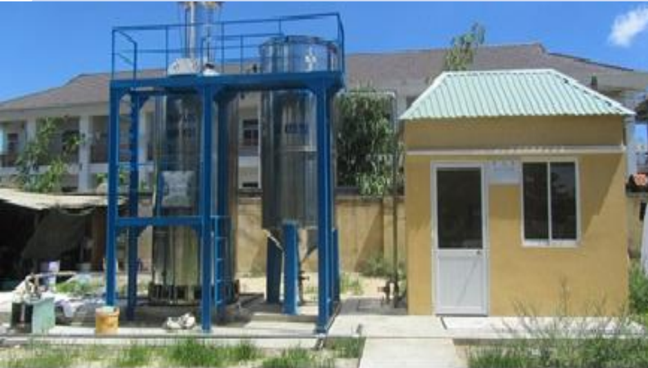
Da Nang Hospital Nursing W.W. treatment system
