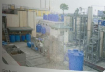
Returned activated sludge Module
