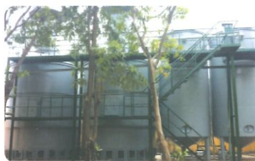
Wastewater treatment plant in Hanoi Milk Joint Joint Stock Company
