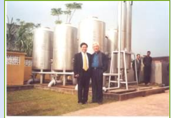
Ground water treatment
