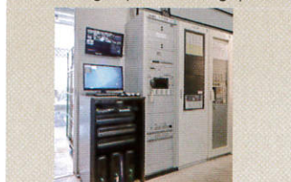
Disaster prevention information receiver and emergency broadcasting system
