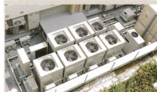
Air-conditioning equipment Air conditioners
