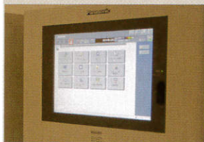
Central monitoring system (WeLBA)
