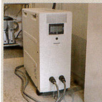
Lithium-ion storage battery system
