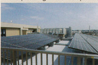
Solar power generation system
