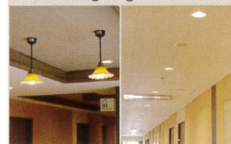
LED lighting fixtures
