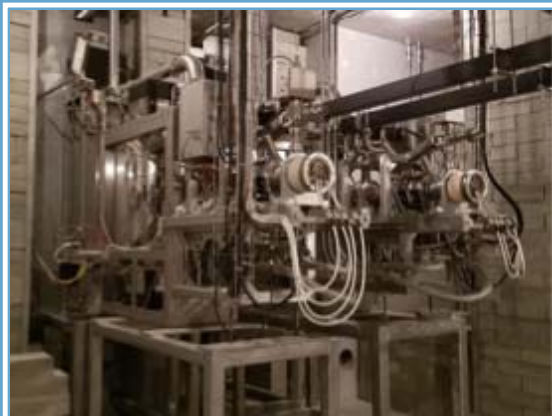
Dual Accelerators (rear view) In Accelerator Room
