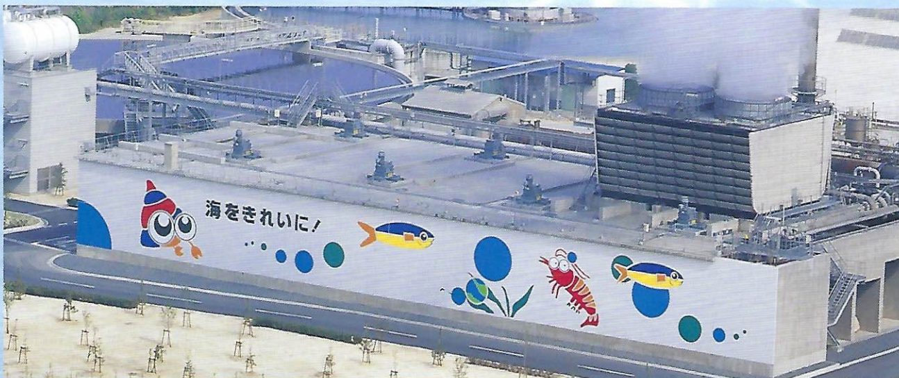
酸素曝気法活性汚泥設備 Activated sludge processing equipment that uses oxygen-based aeration.
