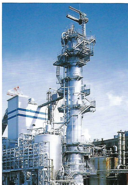
3KP設備 3KP plant
