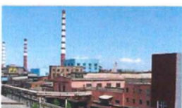
Kazzinc New Metallurgy Waste heat boiler
