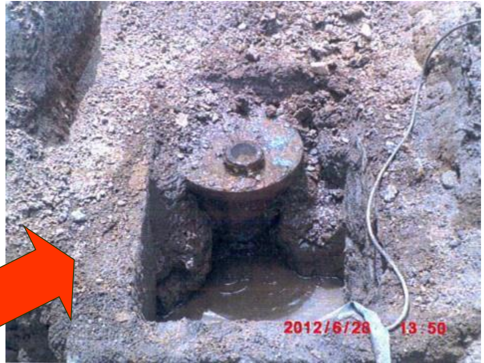
a leaking exhaust valve
