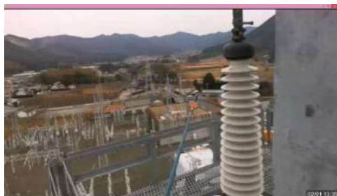
Tower of Transmission line
