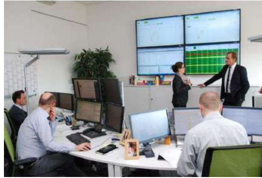
central control room
