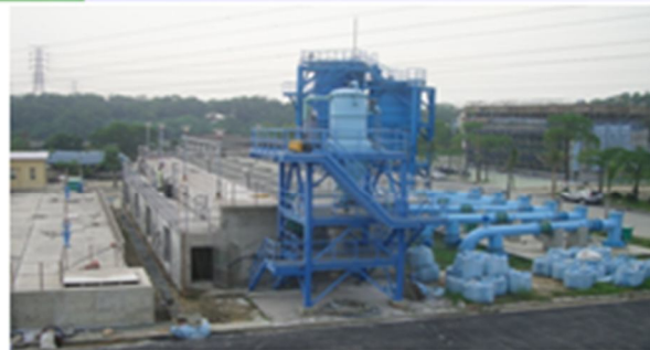
Feng-shan WTP Pellet Softening Facility
