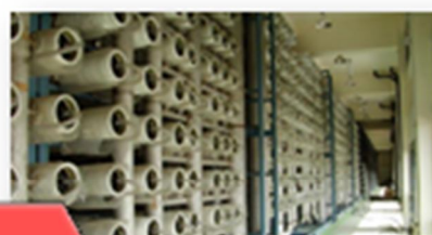
Makong RO Desalination Plant
