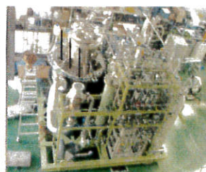
②-1 Hydrogen generator DAINICHI Machine and Engineering
