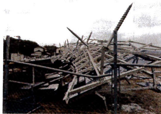
PV panels damaged by the typhoon
