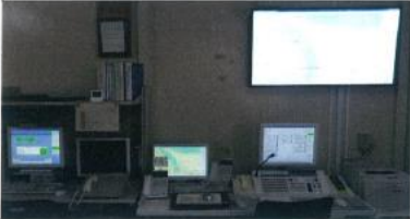
Karatsu City disaster management radio communication network (Broadcast-based communication system and/or mobile communication system) console
