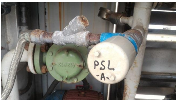
圖 71 Fuel Forwarding SKID 內壓力開關
