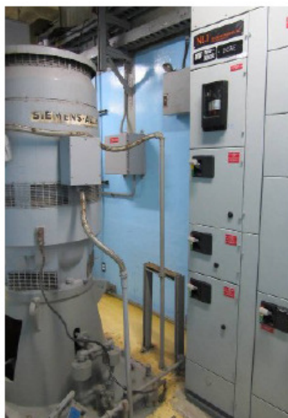
ECW pump and motor (Floor El. 6.6 meter)
