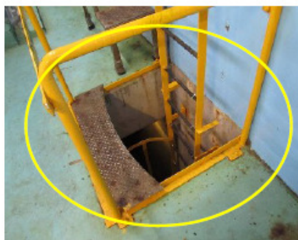
Opening of the ladder (El. 6.6 meter)
