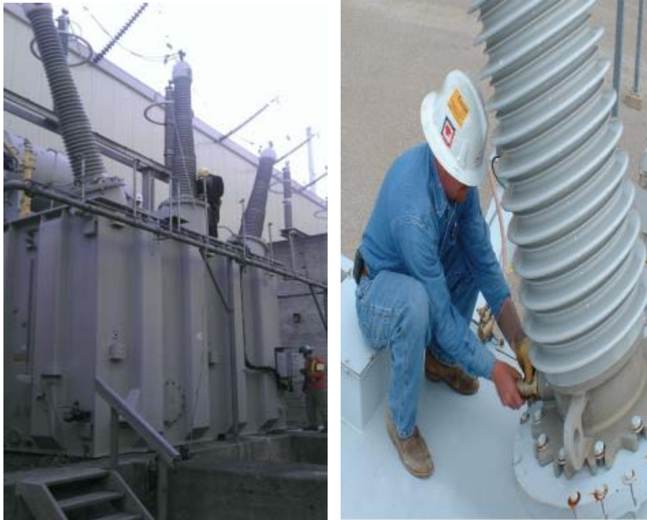
圖 參-37 InsuLogixB installation at BC Hydro Canada. (WEIDMANN)
