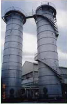
Anaerobic Fluidized Bed the lowest footprint for treating organic wastewater
