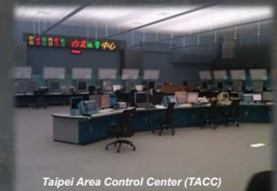
Taipei Area Control Center (TACC)
