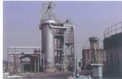
8000 m 3 /d FBC water softening project for Taiwan Water Corporation
