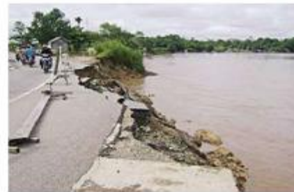
Bank erosion at the Sesayap River in Indonesia
