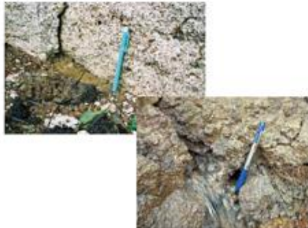
A pipeflow exposed at the head scarp of the landslide is believed to cause slope instability
