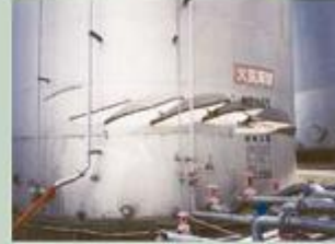
1995年 阪神・淡路大震災で強震動の影響により筒板が変形（座屈）した石油タンク Oil tank with shell plates that deformed (buckled) in response to the strong ground motions during the 1995 great Hanshin-Awaji earthquake
