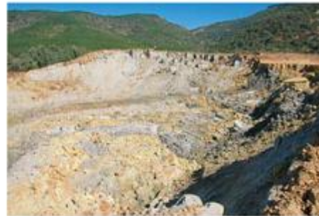
Failure of a tailings dam in Las Palmas, Chile, after the 2010 Chile earthquake
