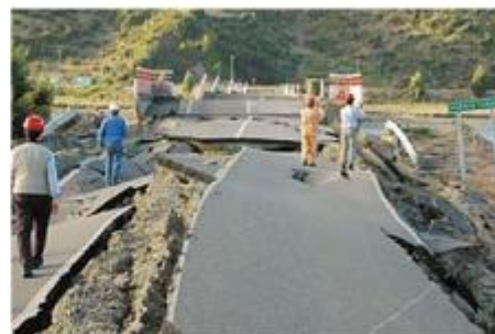
Damaged road embankment at the river mouth of the Rio Tubul after the 2010 Chile earthquake
