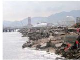
Coastal damage by storm surge and waves
