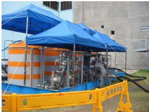
Chemical Injection Pumps
