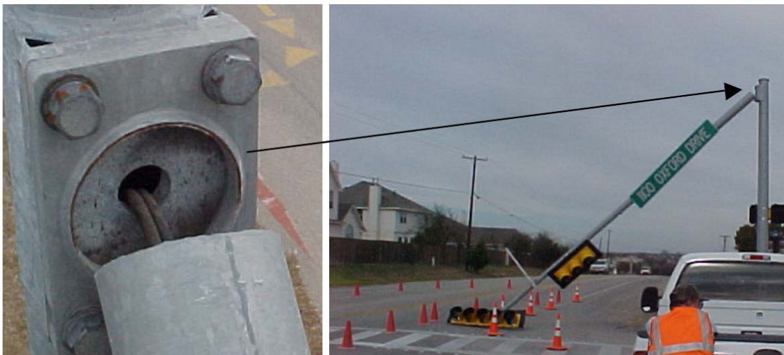
Figure 4. Mast Arm Fatigue Failure
