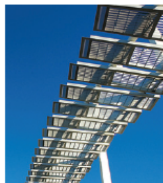
Solar panels at Whitehall Ferry Terminal.
